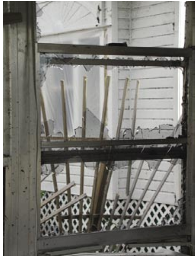
This image dramatically demonstrates the difference in window performance between Liz Hutchinson's home at 311 Taylor Street and her neighbor's home less than 5 feet to the north that did not have security window film.
